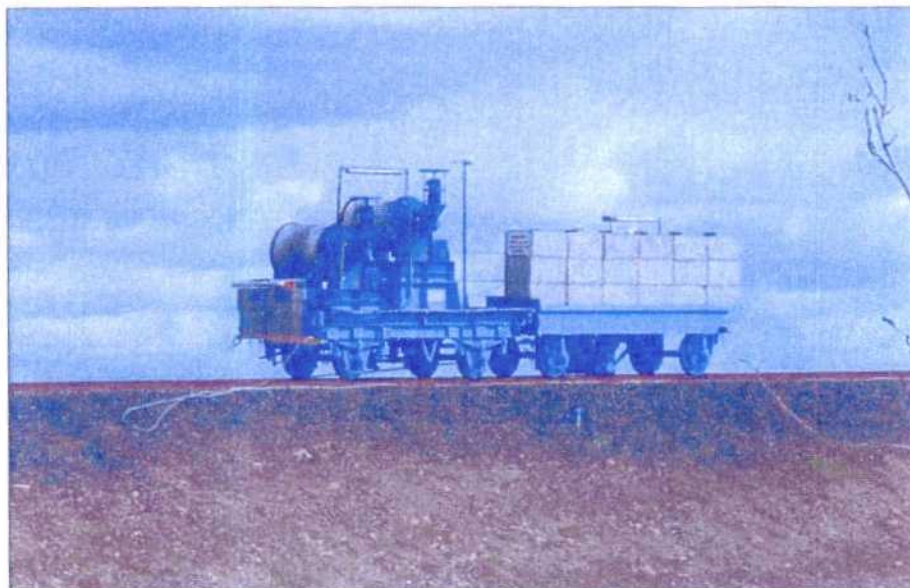
Figure 3.21: Electrically driven winch controlling the tailings distribution pipeline at the Lisheen TMF
